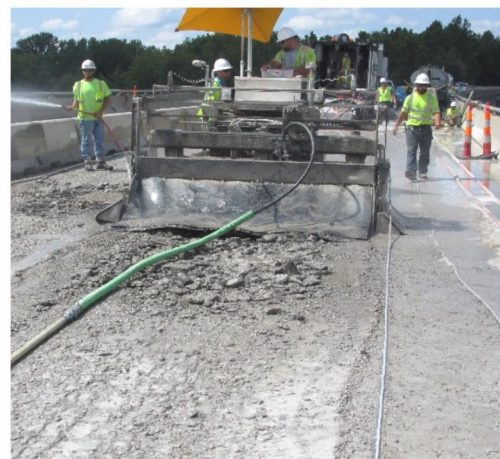
"Fast Track" Hydrodemolition Surface Preparation on the Warsaw Bridge, on Route 7, in Henry County, in 2017. This included 4227 square yards of surface preparation and LMC overlay.
